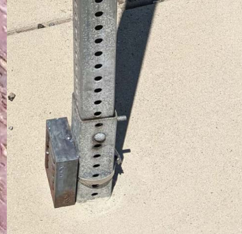
← Heat sensor installed on a street sign.
